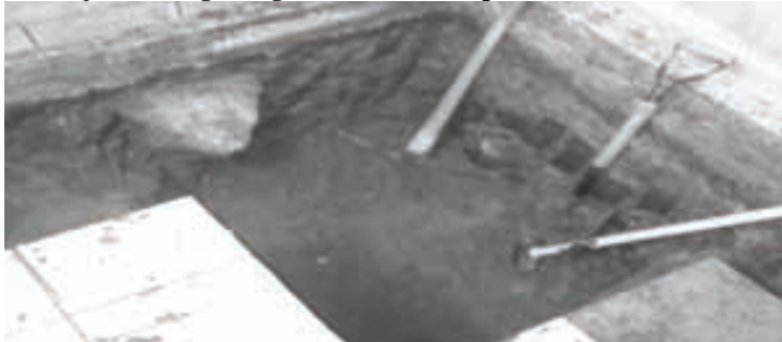
Photographed here is the corner under the east stair case leading to the Parish hall that will hose drainage pipes leading from the sump pump under the same stair case out to the internal storm system to be installed in our parking lot that will eventually connect to the Town of Richmond Hill storm system
