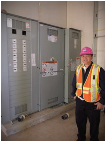
Fr. Arthur Amian visits the construction site and admires the huge electrical panels that were recently installed.
