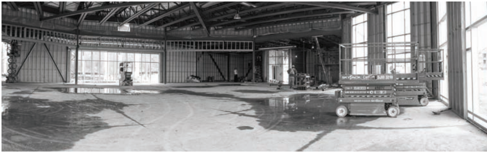
Our future parish hall which will sit about 400 people auditorium style, thanks to your continued financial support to our Building Fund
