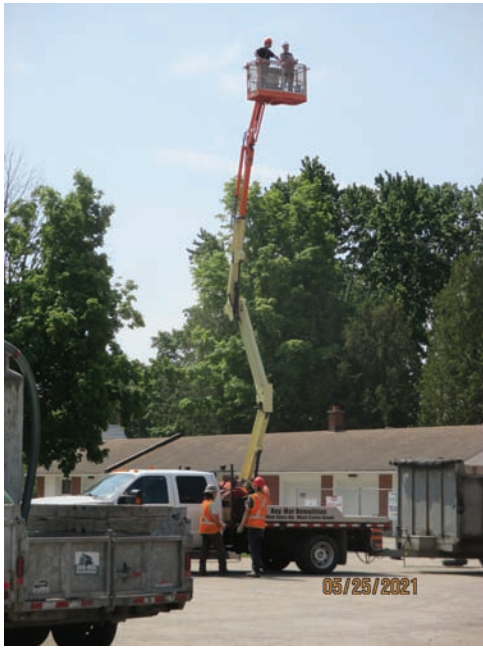
Fr. Kuzma getting a bird's eye view of the demolition project this week.
